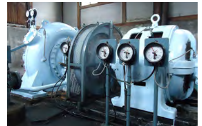
Hiroshima Gas Shiwahori Power Station (small-scale hydropower generation)
