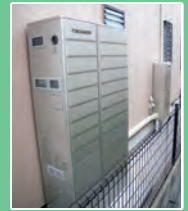
Kitchens, hot water supply, etc.
