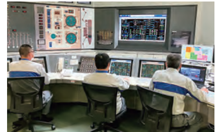
Central control room
