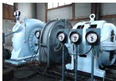
Hiroshima Gas Shiwahori Power Station (small-scale hydropower generation)
