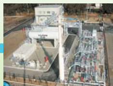
Mizushima station (Setouchi Pipeline Co., Ltd.)
