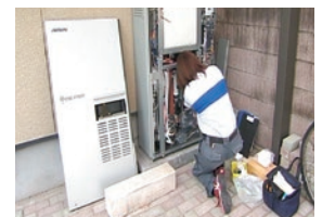
Maintenance of an "Ene-Farm" household fuel cell
