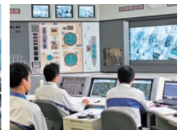
Central control room
