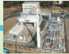
Mizushima station (Setouchi Pipeline Co., Ltd.)
