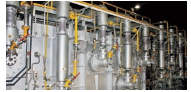
Gas industrial furnace
