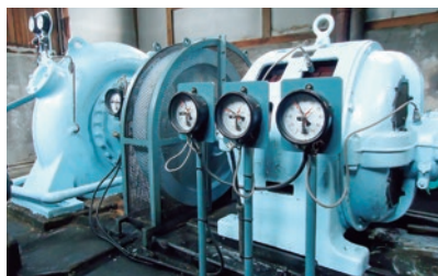
Hiroshima Gas Shiwahori Power Station (water turbine and generator)
