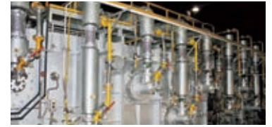
Gas industrial furnace
