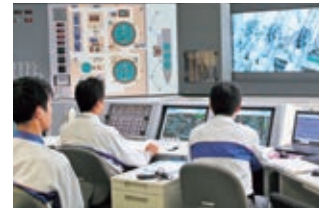
Central control room
