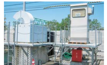
Power generation system based on differential gas pressure
