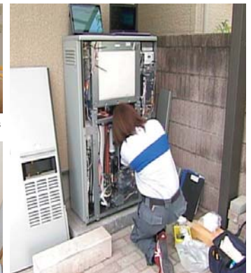
Maintenance of an "Ene-Farm" household fuel cell
