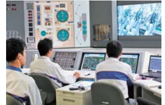
Central control room
