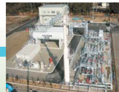
Mizushima station (Setouchi Pipeline Co., Ltd.)
