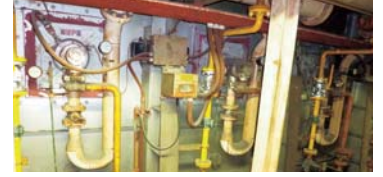
Gas industrial furnace
